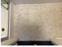
Damaged and dented floor
