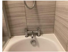
Water stain near taps
