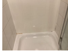
Mould above sealant.
