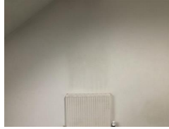
Stain above radiator
