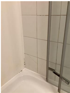
Cracked shower tile
