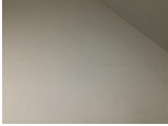
Light wall stains
