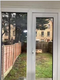
PVC frame slightly discoloured on top
