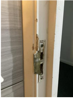
Damaged door frame
