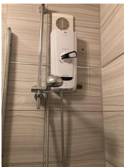
Damage next to control panel. Dirty extractor fan
