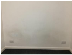
Heavier staining and damage to paint
