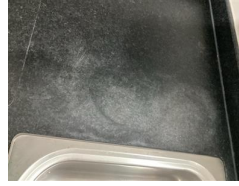
Stains on counter top next to wash basin.
