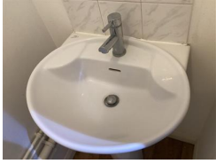
Dirty mouldy wash basin
