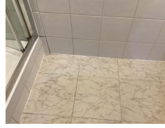
Dirty grouting and loose tiling
