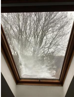
Condensation or blown window glass. Rotting frame
